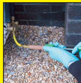
Fluorescent dye is added to the system
