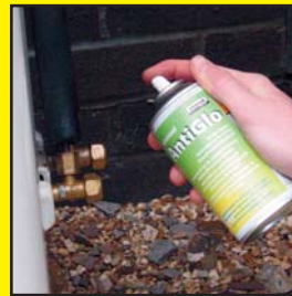
Once repaired residual dye is removed from leak sites.
